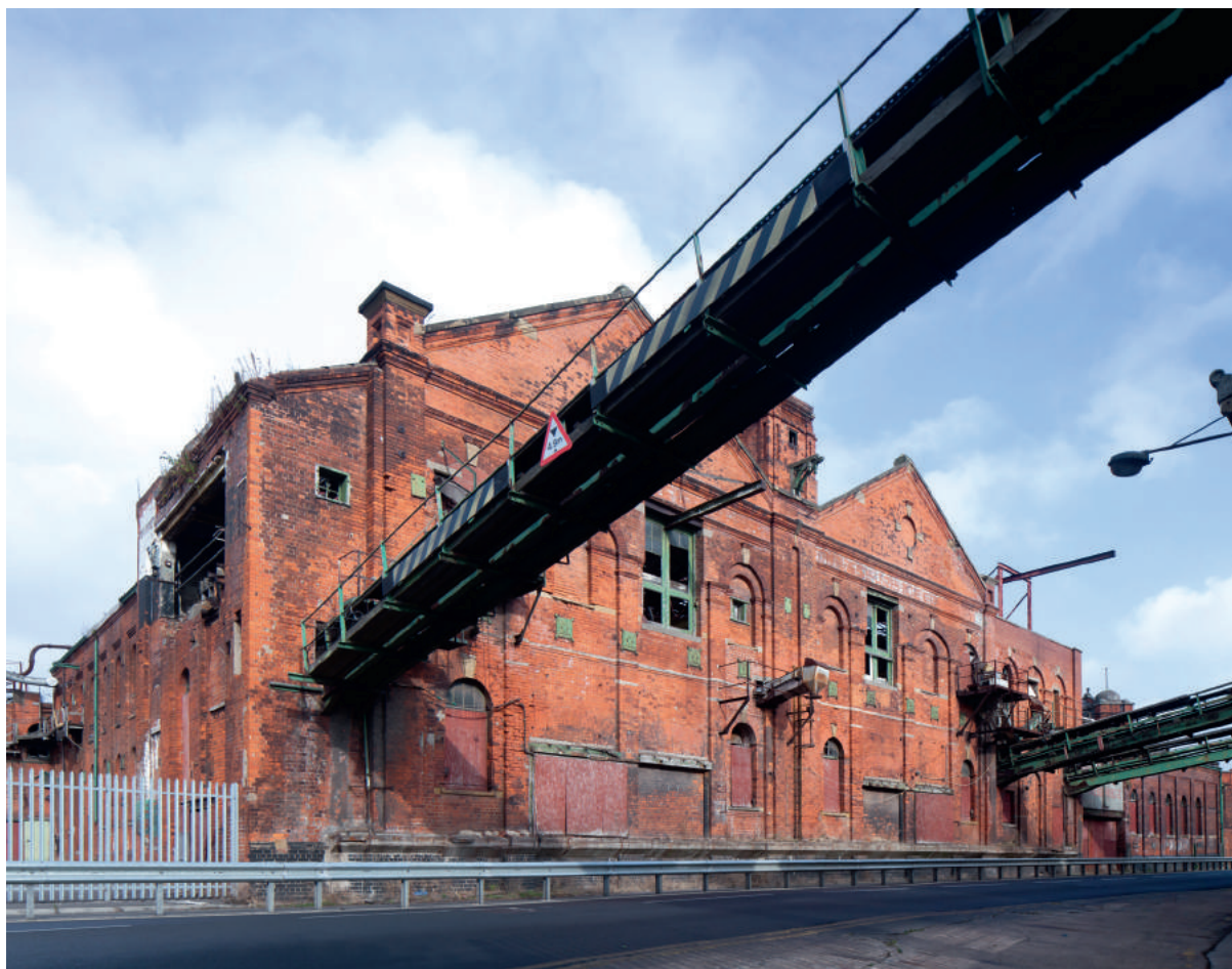
The vast Grimsby Ice Factory, built in 1900–1, empty and in a serious state of decay. Image: Andy Marshall
