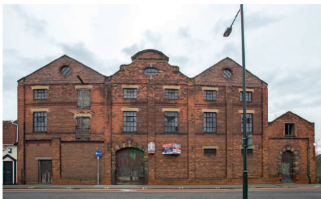
Hewitts Brewery in Grimsby, featured in the 2017-18 Buildings at Risk catalogue. Image: Eveleigh Photography
