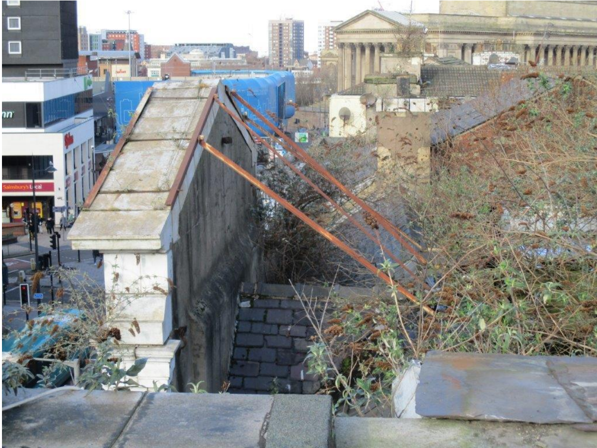
Photograph 5: Restraint straps to pediment
