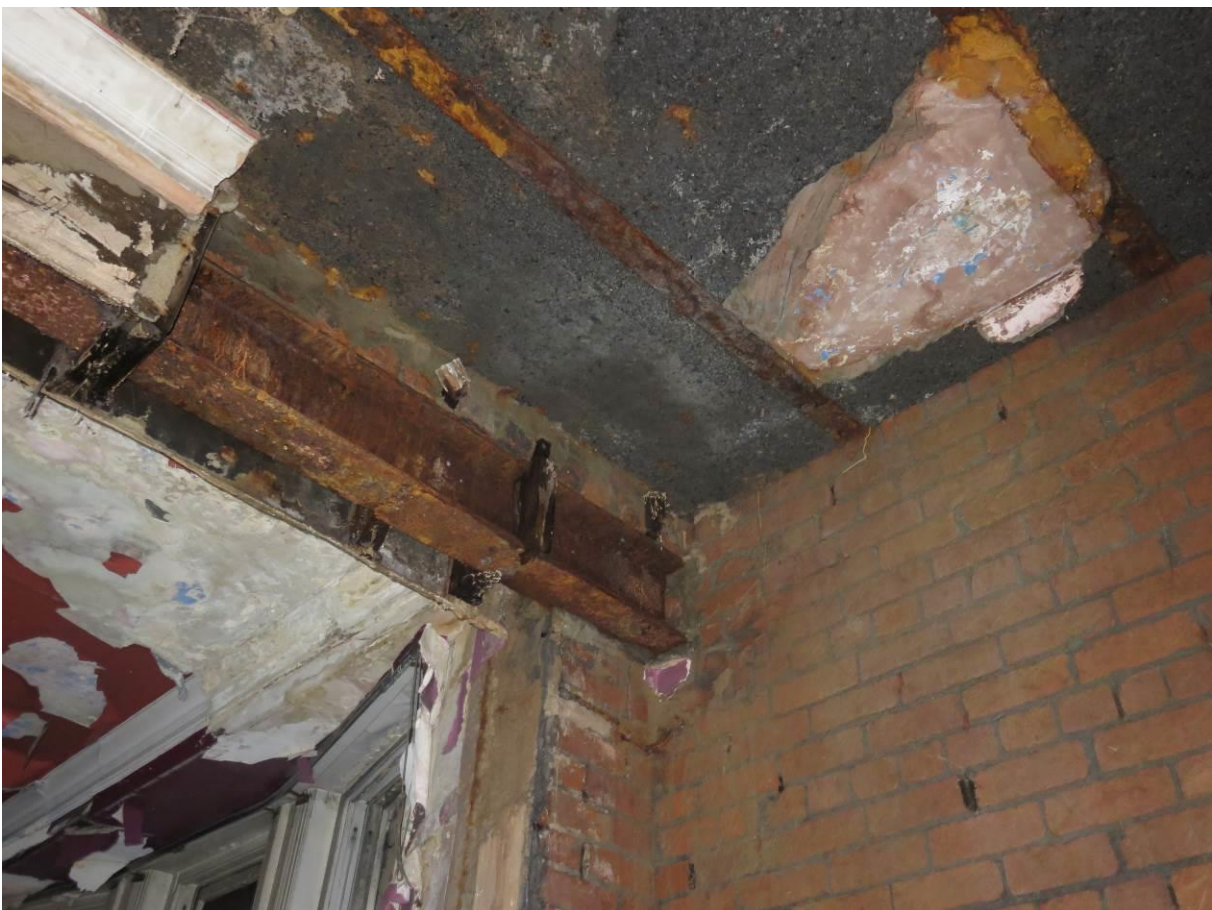
Photograph 4: Steel beam to front elevation with no evidence of corrosion jacking to built-in end
