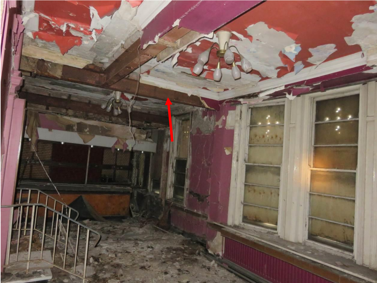
Photograph 3: First floor room with steel beams spanning front elevation back to the cross wall behind
