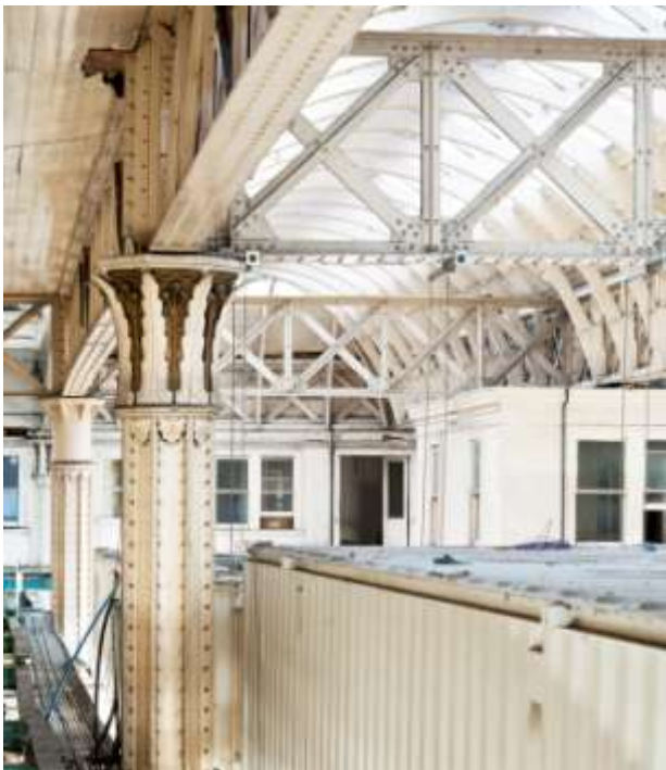
The impressive engineering work inside the General Market, including ornate Phoenix Columns
