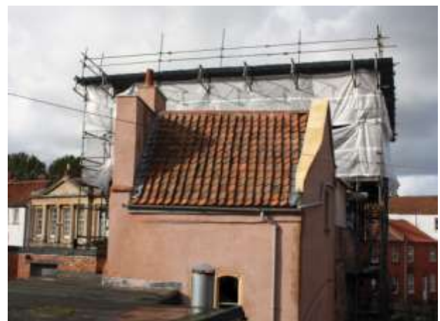
The back of Castle House, Bridgwater, that has been partially repaired by the SAVE Trust.
