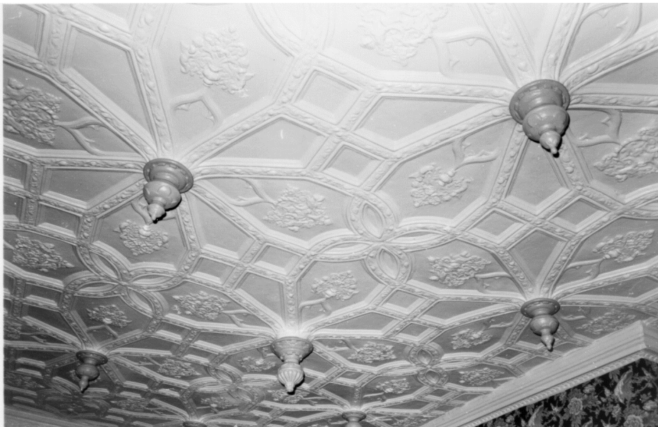
Small Street, no 15, detached parlour block to the rear, ceiling of the early 17th century, photograph of 1979 (RHL)
