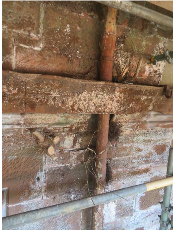
Photograph 44: Defective downpipe extending through fake 'stone hopper'
