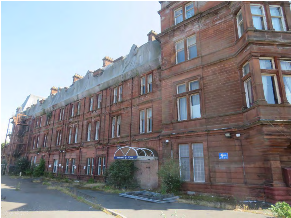
Photograph 95: Vegetation growth to west elevation of North Range
