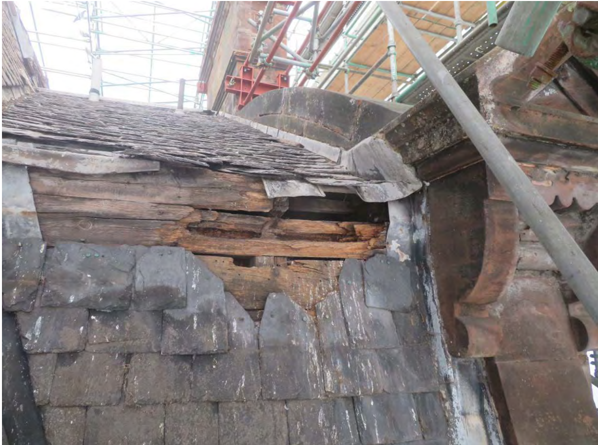
Photograph 22: Local decay to roof structure through water ingress to east elevation
