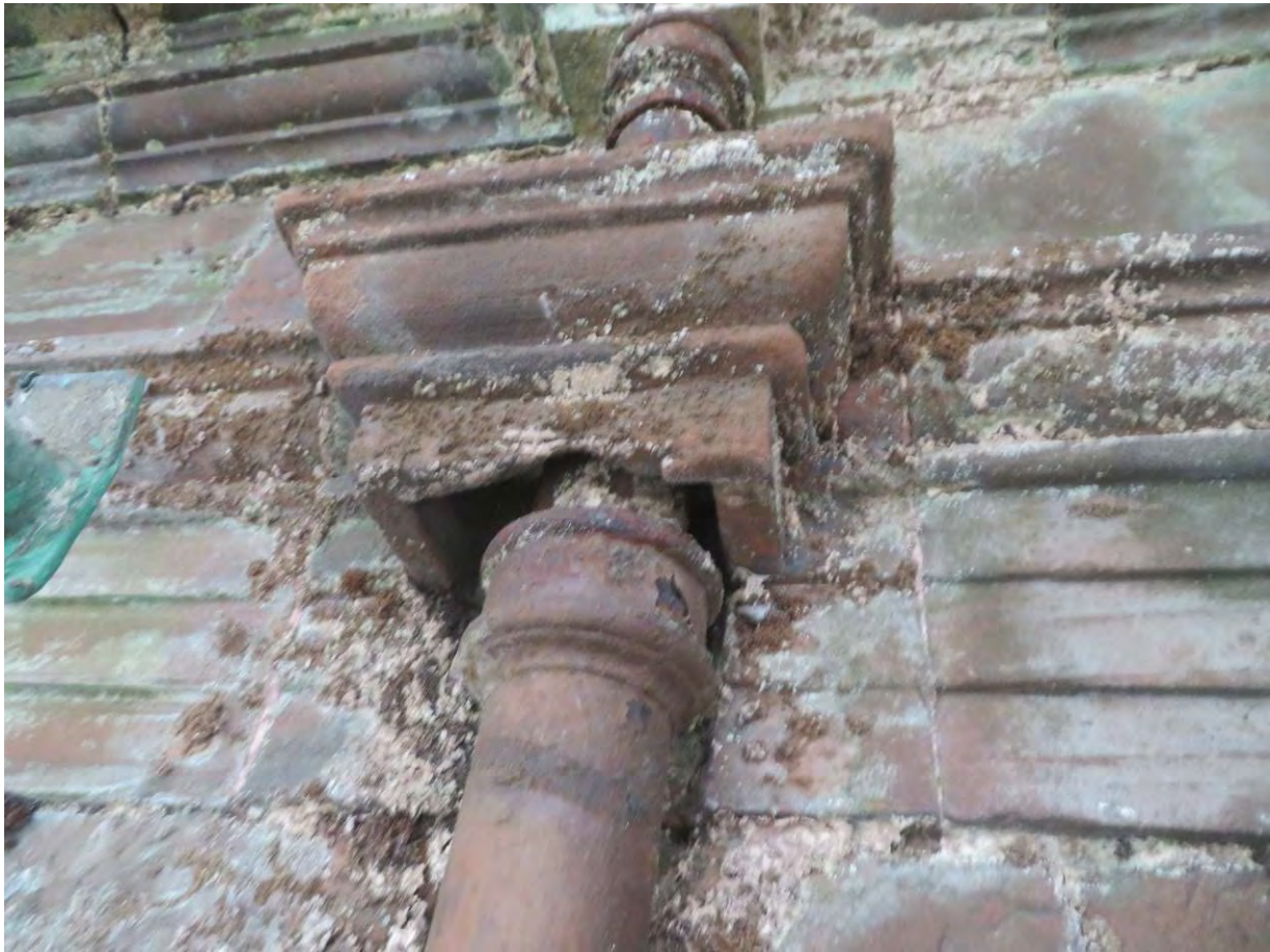
Photograph 45: Fake 'stone hopper' and defective downpipe
