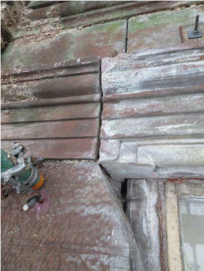
Photograph 47: Loss of stone due to root action of woody shrub above
