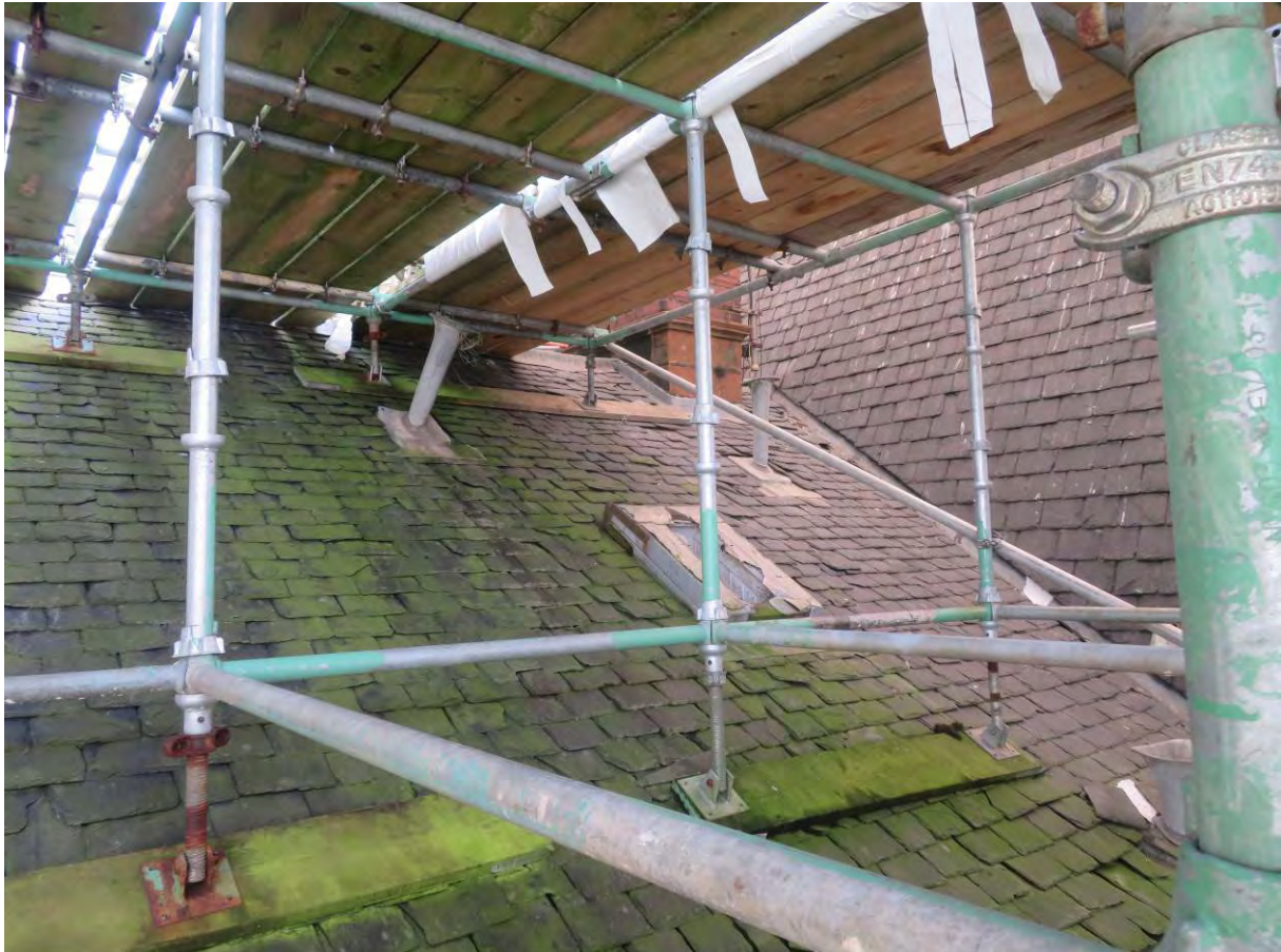
Photograph 88: Roof to dog-leg between Tower and South Range to south side
