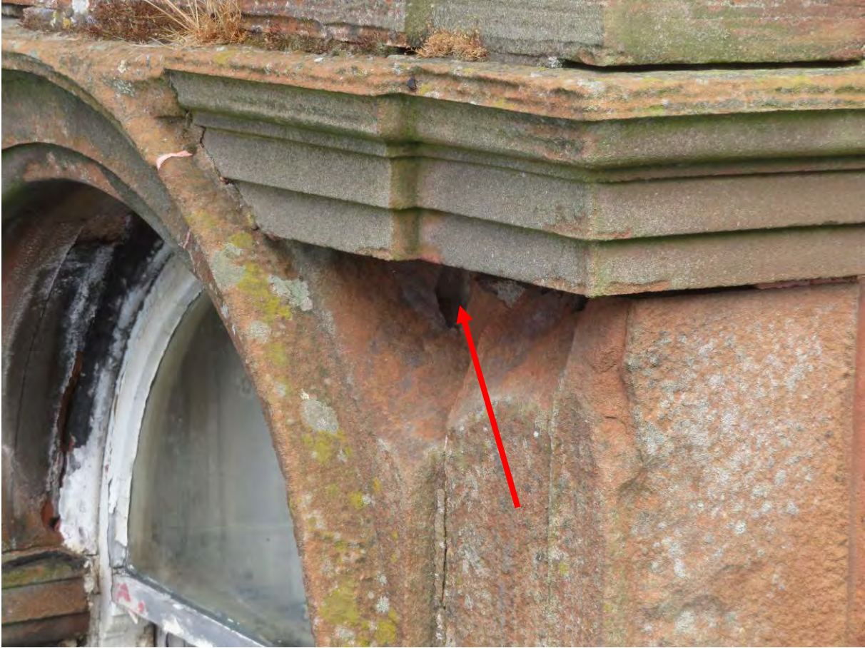
Photograph 84: Potential corroding fixing position
