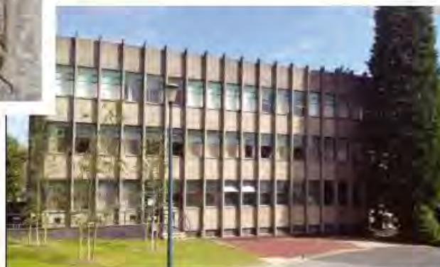
FIGURE 6: Major structural defects were uncovered at George Green Library, University of Nottingham
