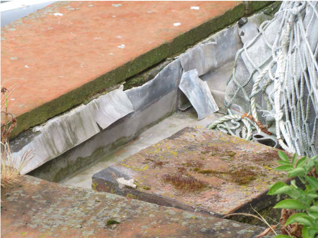
Photograph 83: Loose flashings to tower roof
