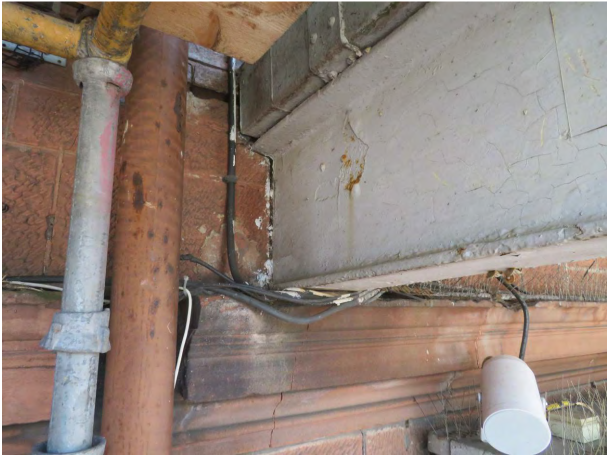
Photograph 59: Main station beam with apparent corrosion jacking to end
