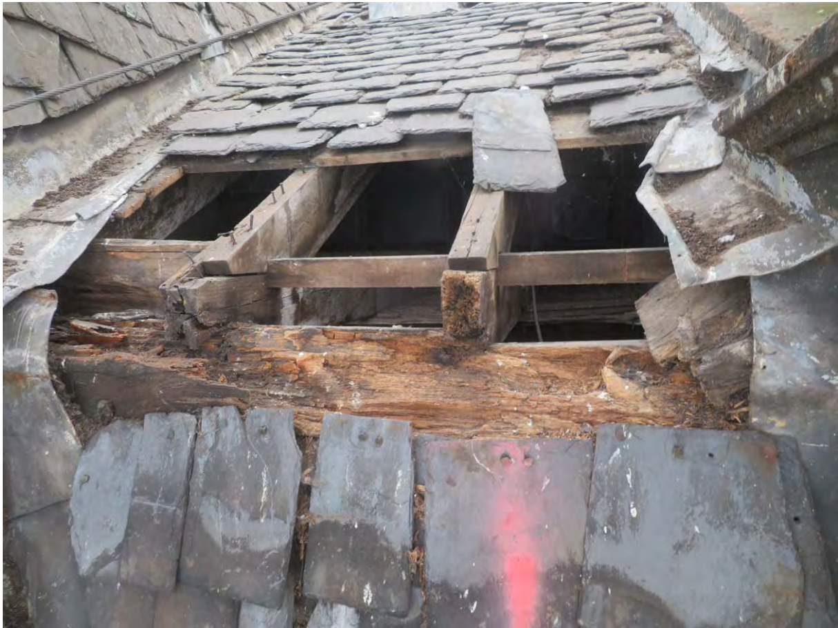
Photograph 19: Local decay to roof structure through water ingress to east elevation
