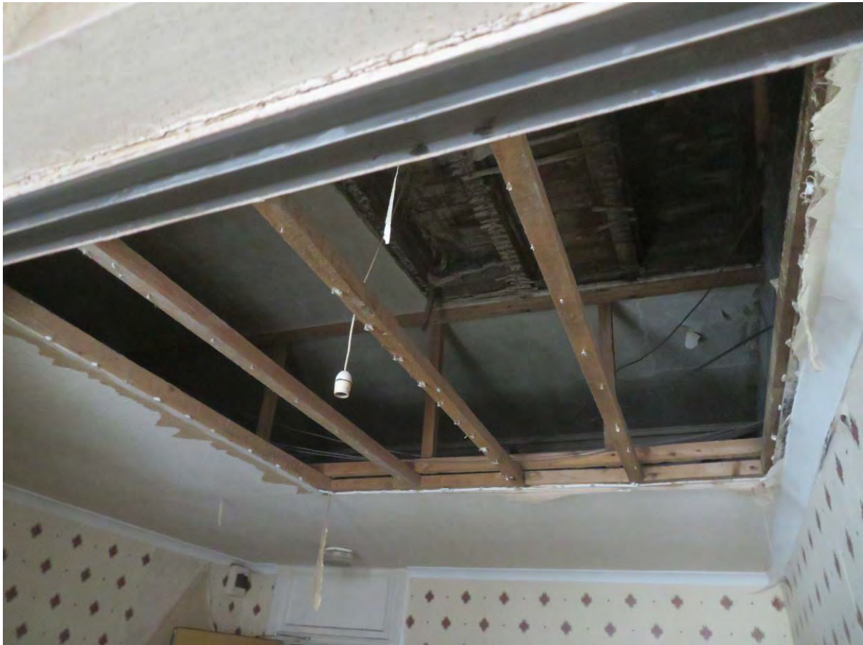
Photograph 73: Main floor joists visible where section of lath and plaster lost
