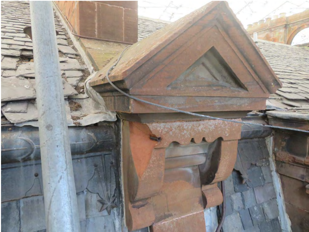
Photograph 41: Damaged stone from old scaffold fixing
