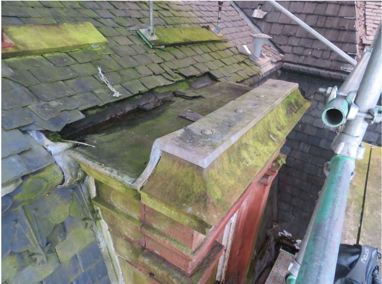
Photograph 90: Head of dormer to dog-leg roof to south side
