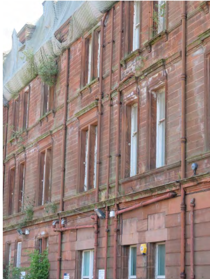
Photograph 96: Vegetation growth to west elevation of North Range
