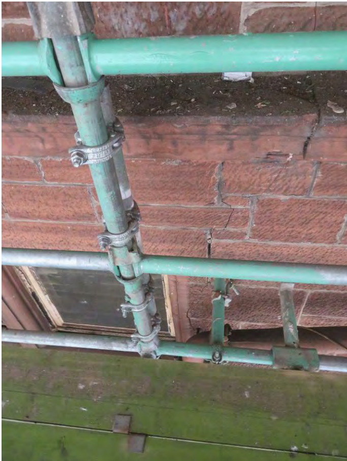
Photograph 57: Movement cracks to north east corner
