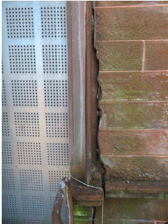
Photograph 99: Cracking to door reveal from fire escape
