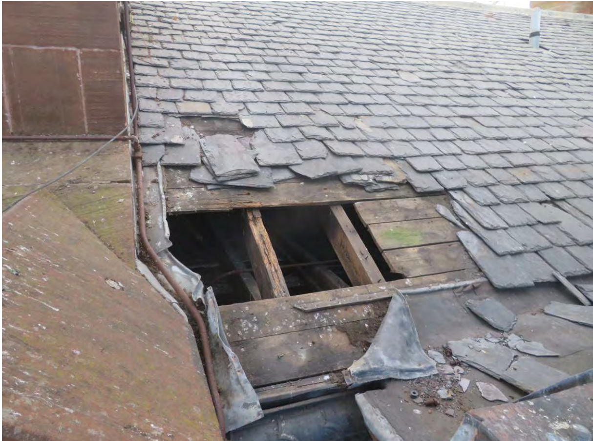
Photograph 18: Local decay to roof structure through water ingress
