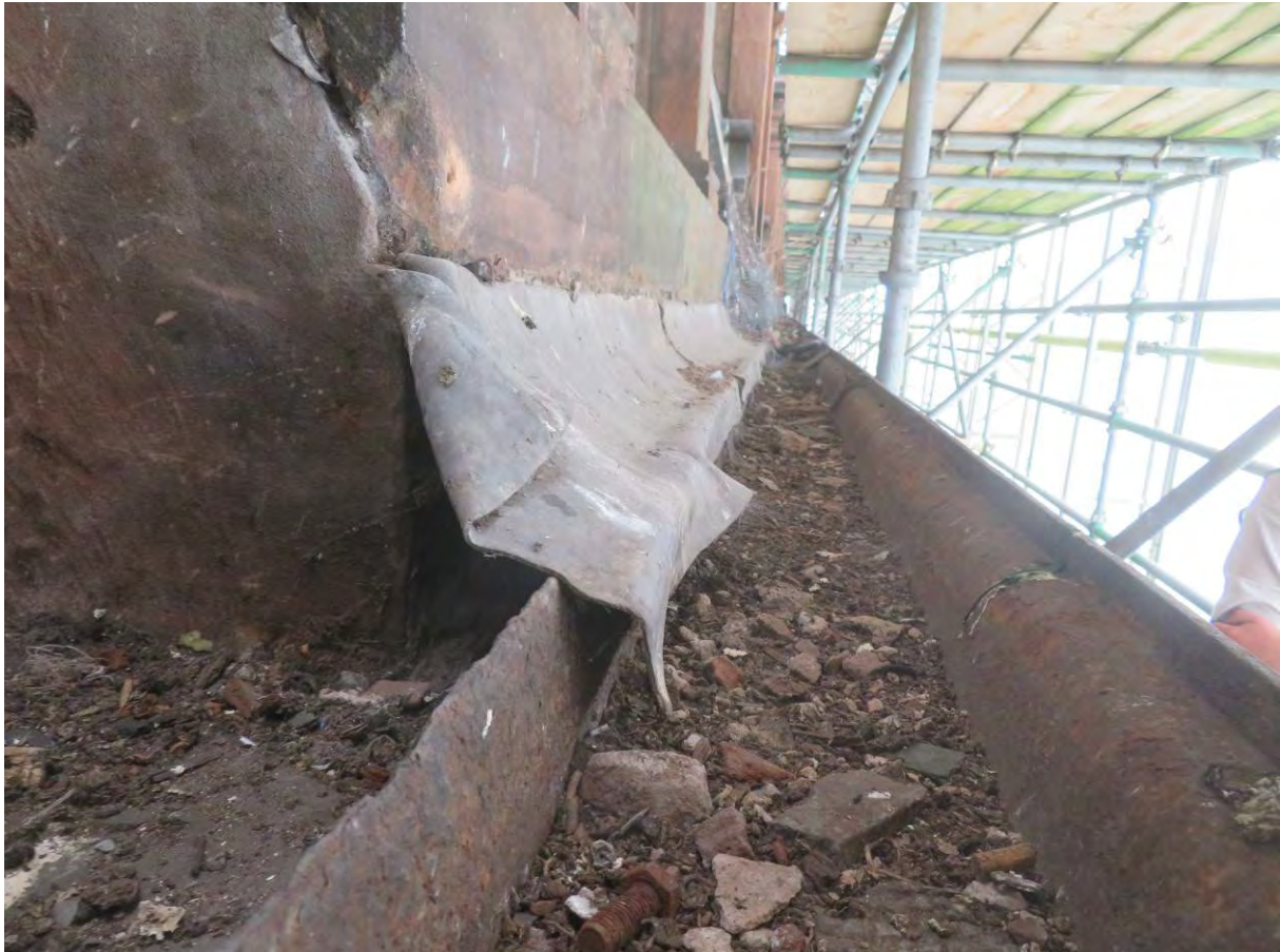
Photograph 34: Cast iron gutter at base of mansard
