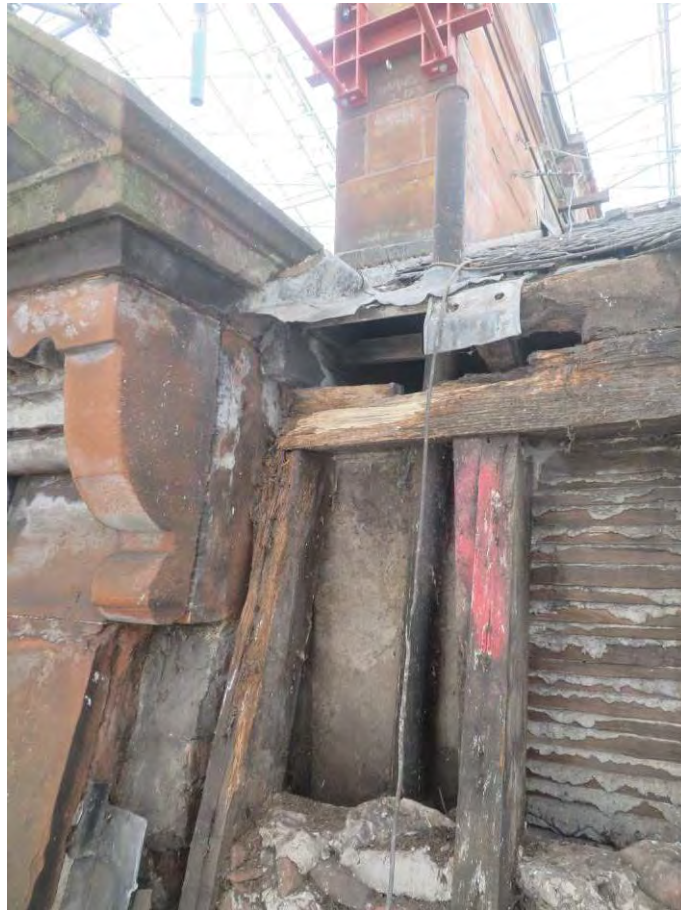
Photograph 21: Local decay to roof structure through water ingress to east elevation
