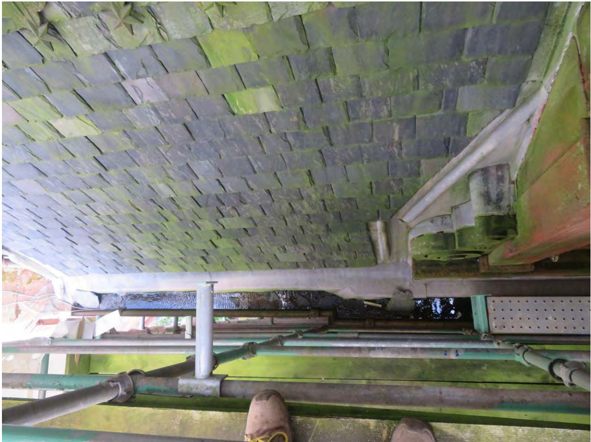
Photograph 89: Standing water in gutter
