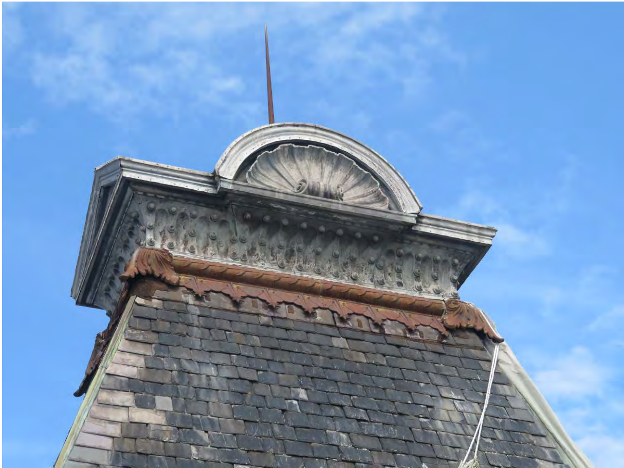
Photograph 81: Head of tower with cast iron decorative weathering
