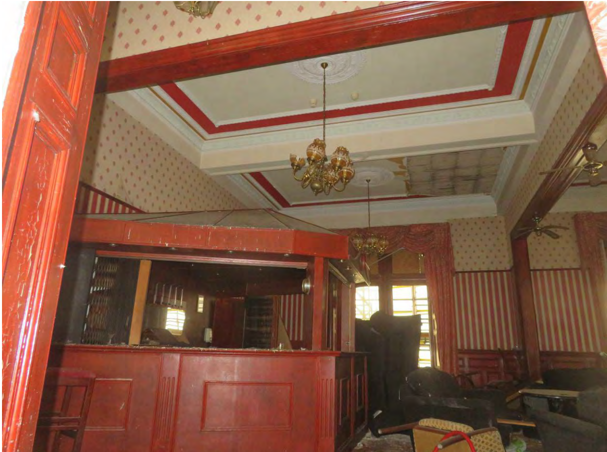
Photograph 76: Principal room with ceiling in reasonable condition but some plaster loss
