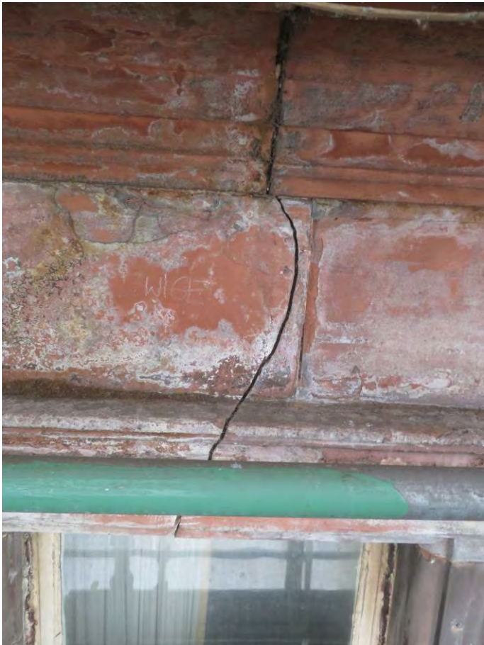
Photograph 39: Fracture to window head
