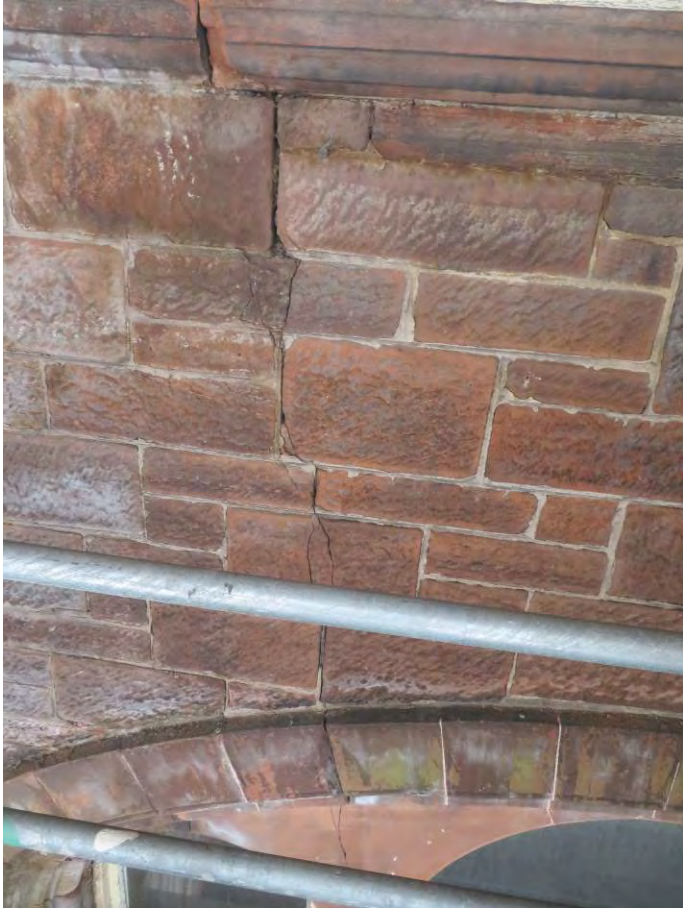
Photograph 58: Movement cracks to north east corner
