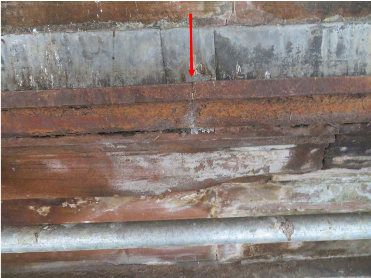
Photograph 35: Damage to stone below gutter joint
