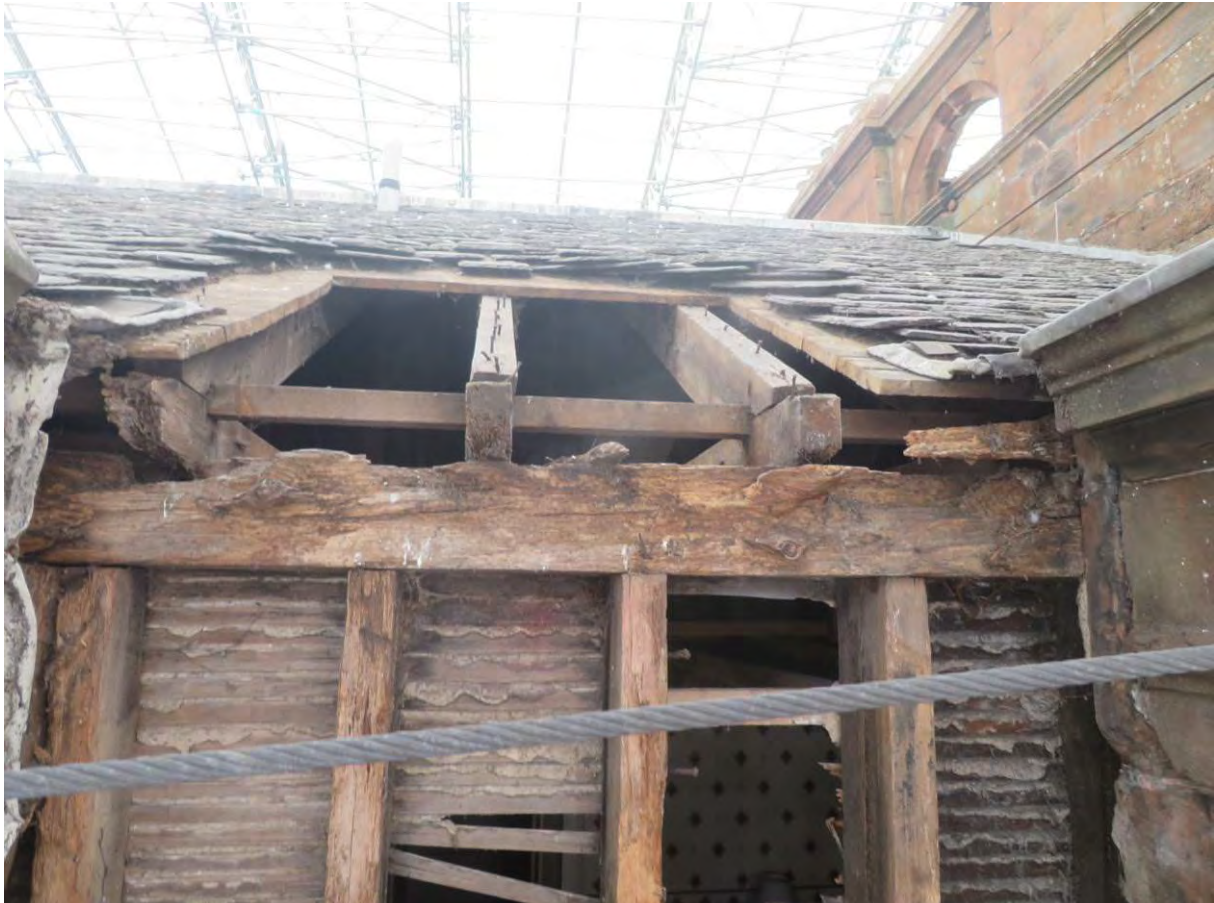
Photograph 20: Local decay to roof structure through water ingress to east elevation
