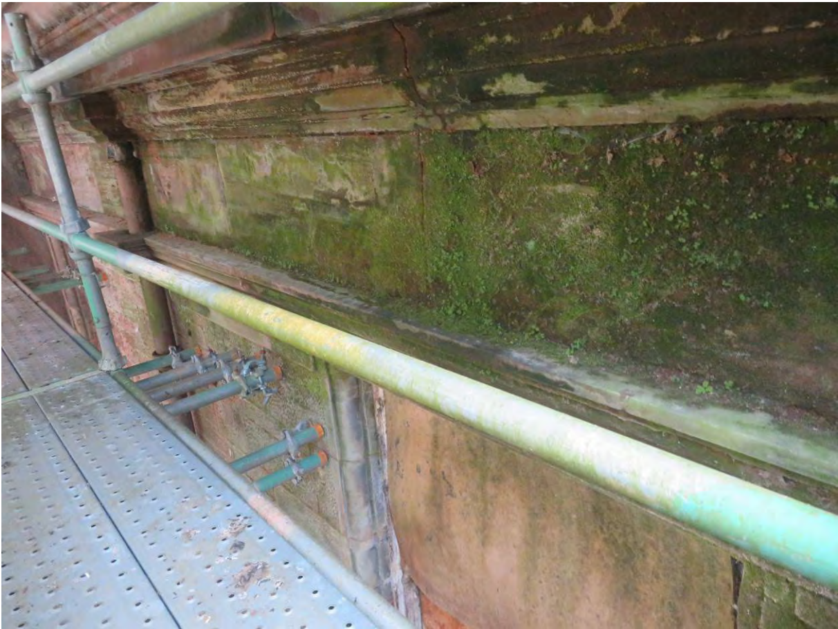
Photograph 55: Significant moisture to west end of north elevation
