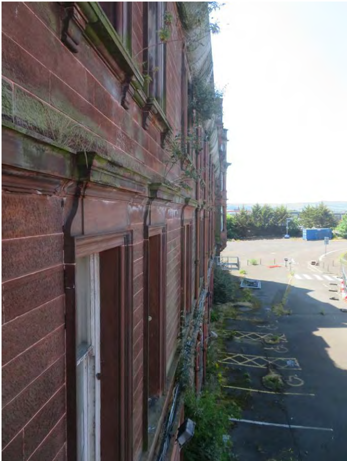
Photograph 97: Vegetation growth to west elevation of North Range
