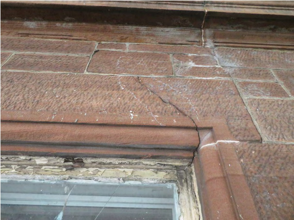
Photograph 40: Fracture to window head
