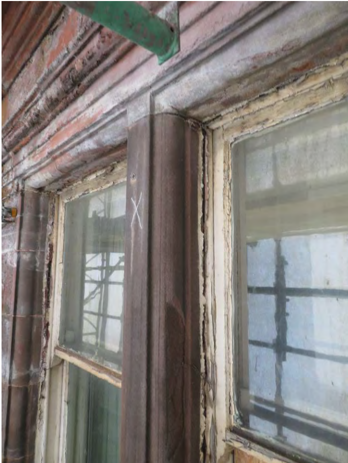
Photograph 50: Failed face of stone mullion
