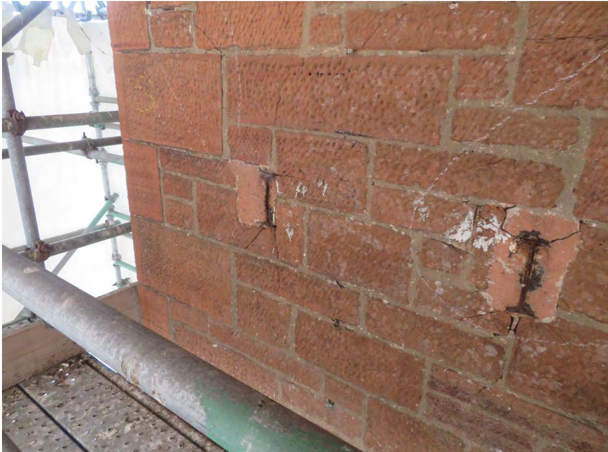
Photograph 42: Steel or iron beams built in and corroding causing damage to stone
