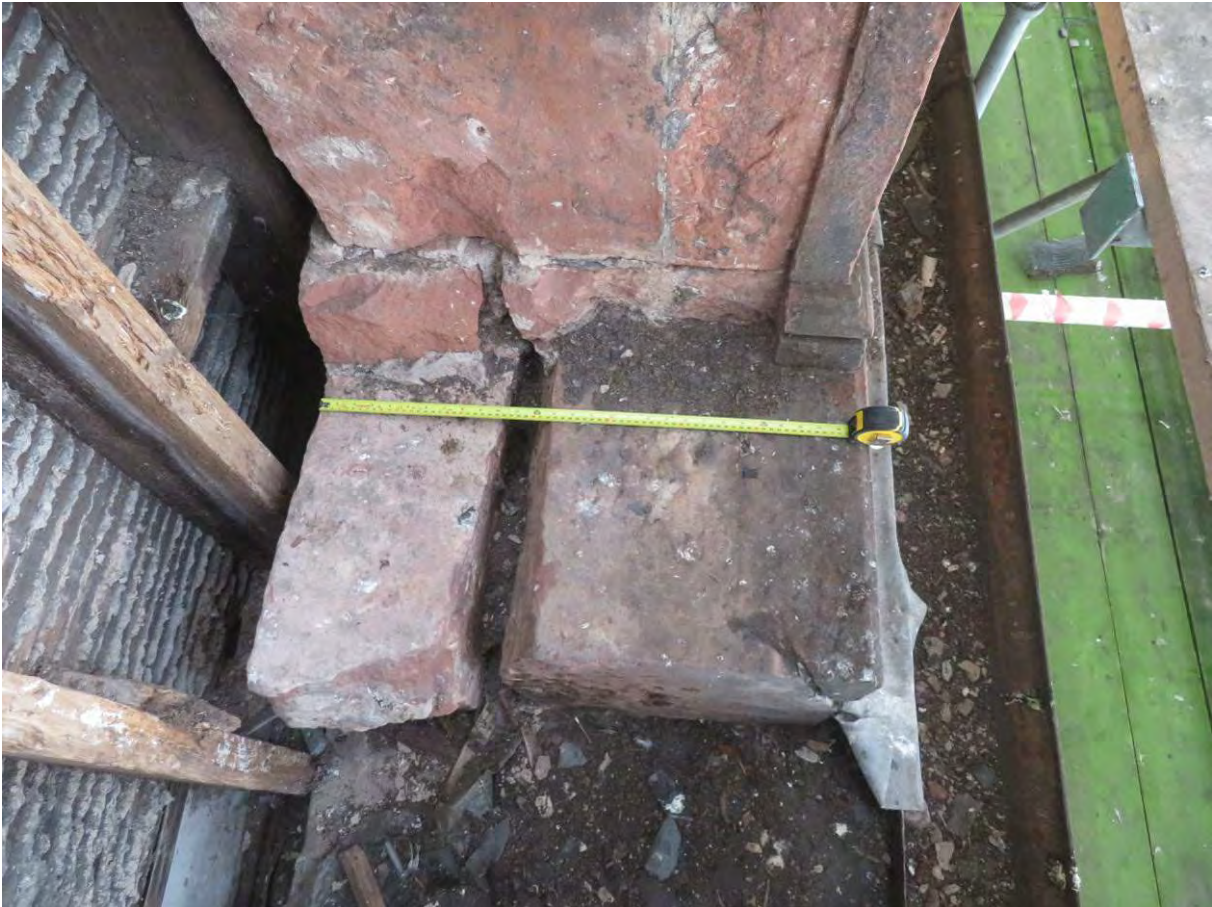
Photograph 28: Wall thickness at position where dormer exposed to east elevation
