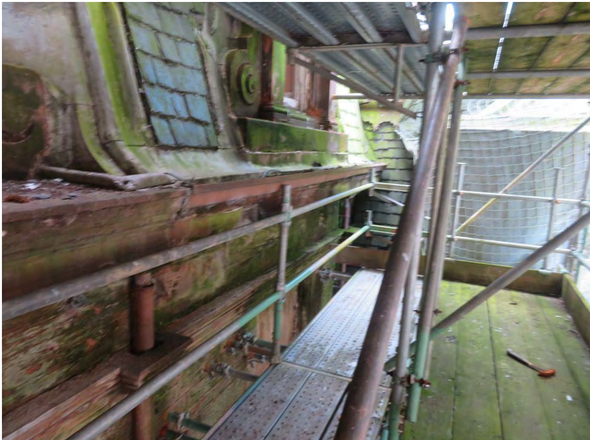
Photograph 54: Significant moisture to west end of north elevation
