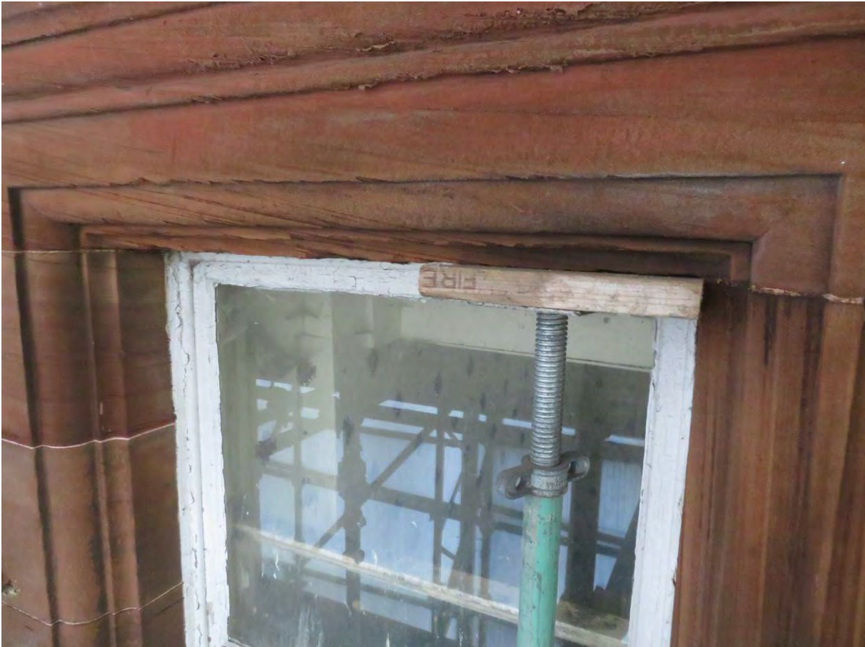
Photograph 52: Prop to eroded window head
