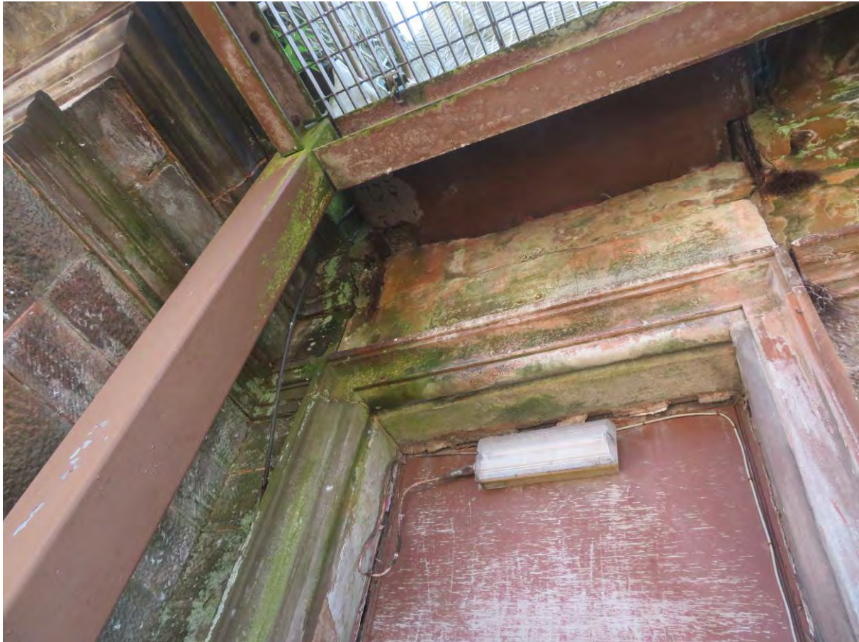
Photograph 100: In-built steel causing stone damage where corroded
