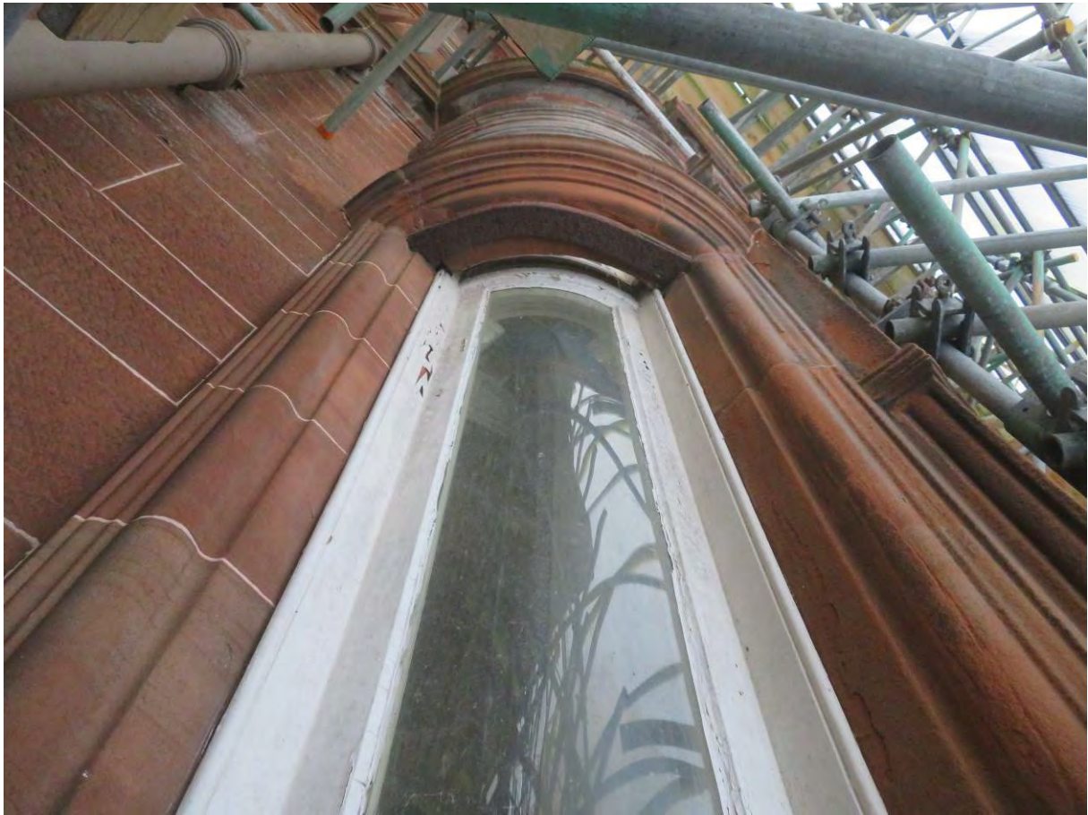
Photograph 65: Steel or iron plate below fractured lintel
