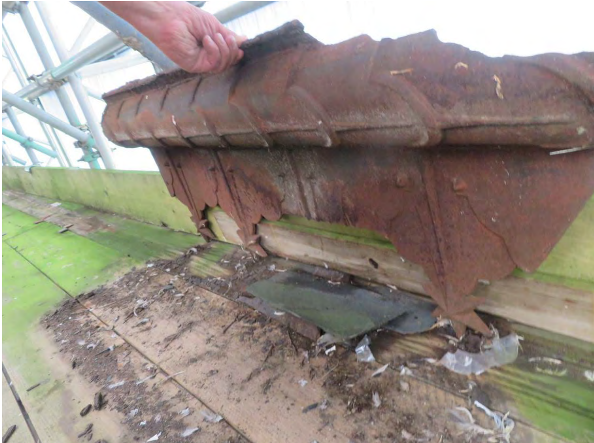
Photograph 24: Broken section of cast iron weathering
