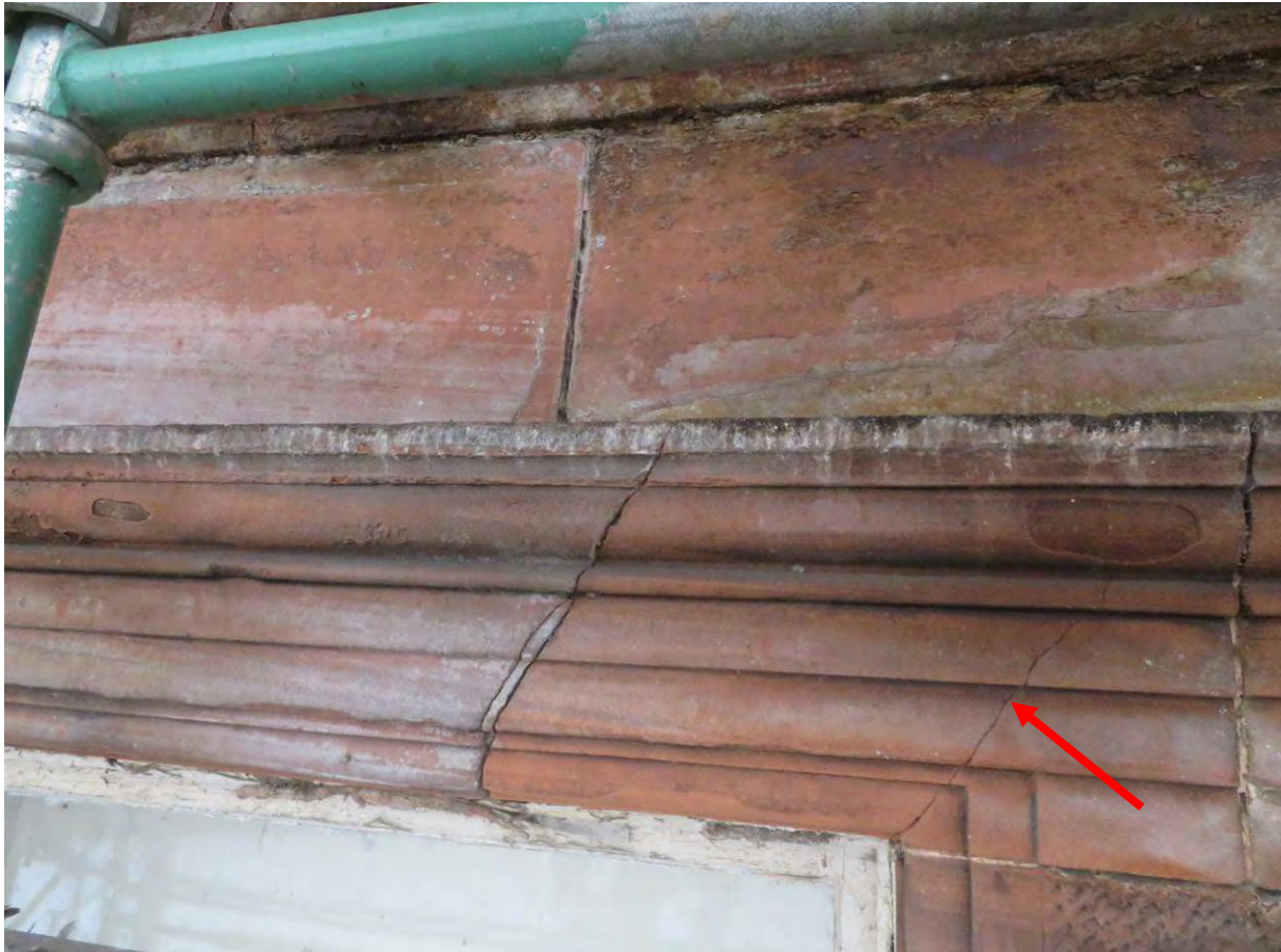
Photograph 38: Fracture to window head
