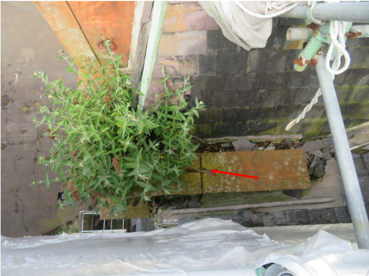
Photograph 85: Cramp to copings
