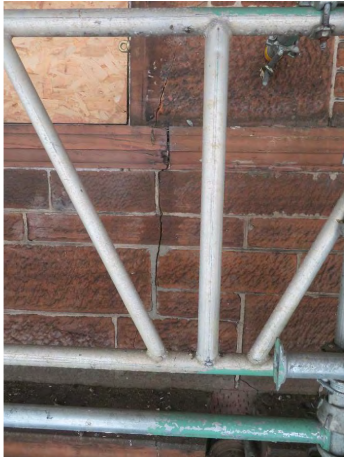
Photograph 56: Movement cracks to north east corner
