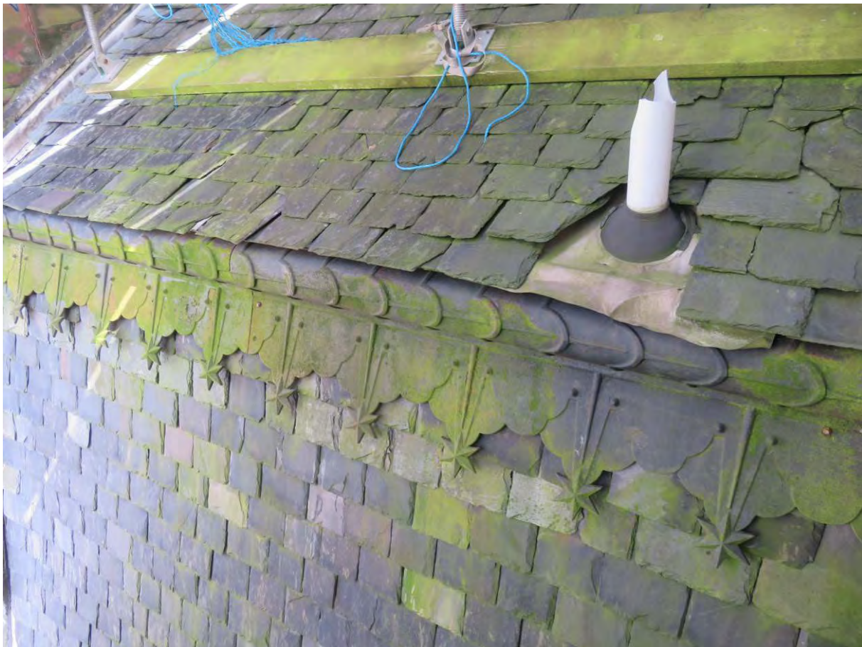
Photograph 23: Cast iron weathering between roof pitches to south range mansard
