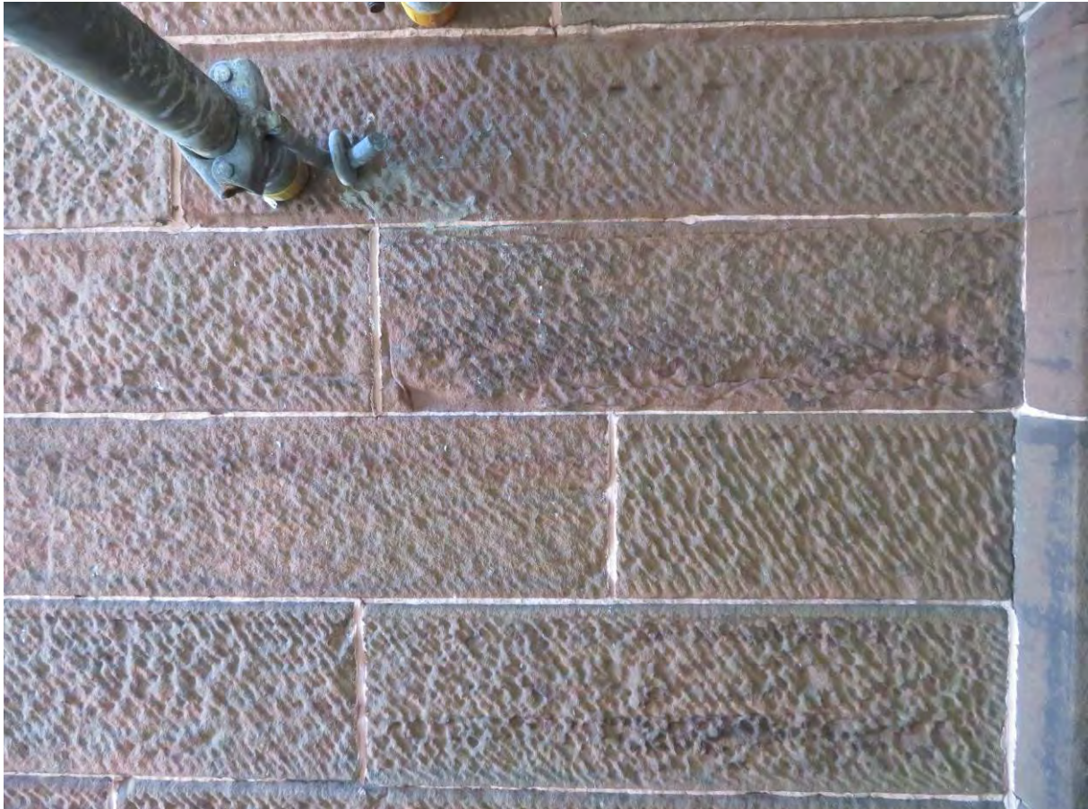
Photograph 62: Tight and possibly lime putty joints to public facing elevations
