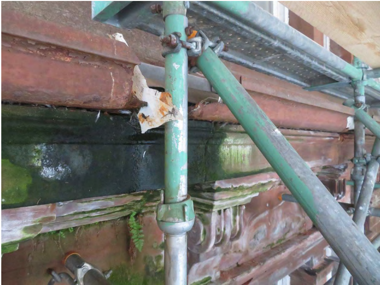
Photograph 61: Significant damp and current water damage
