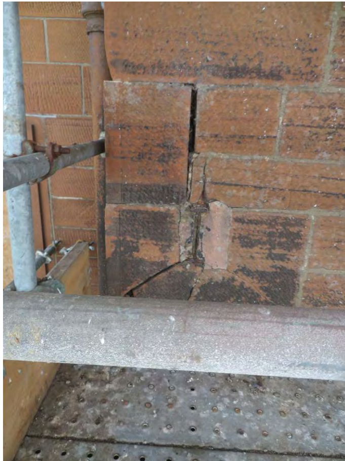
Photograph 43: Steel or iron beams built in and corroding causing damage to stone
