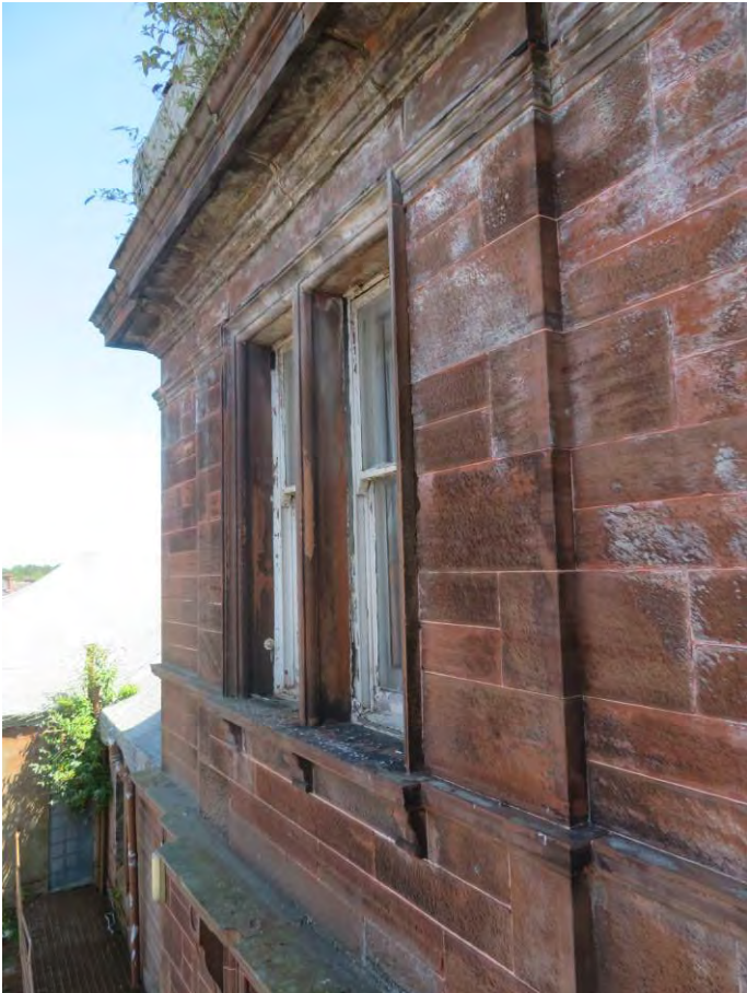
Photograph 98: Vegetation growth to west elevation of North Range
