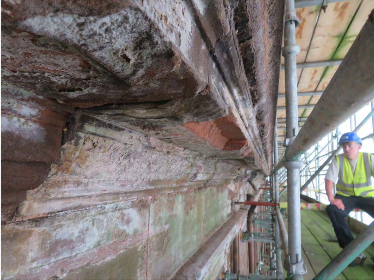
Photograph 36: Damage to stone below defective gutter
