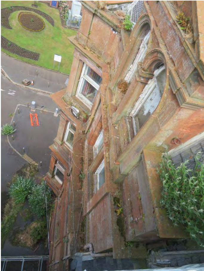
Photograph 86: Windows to tower in relatively poor condition
