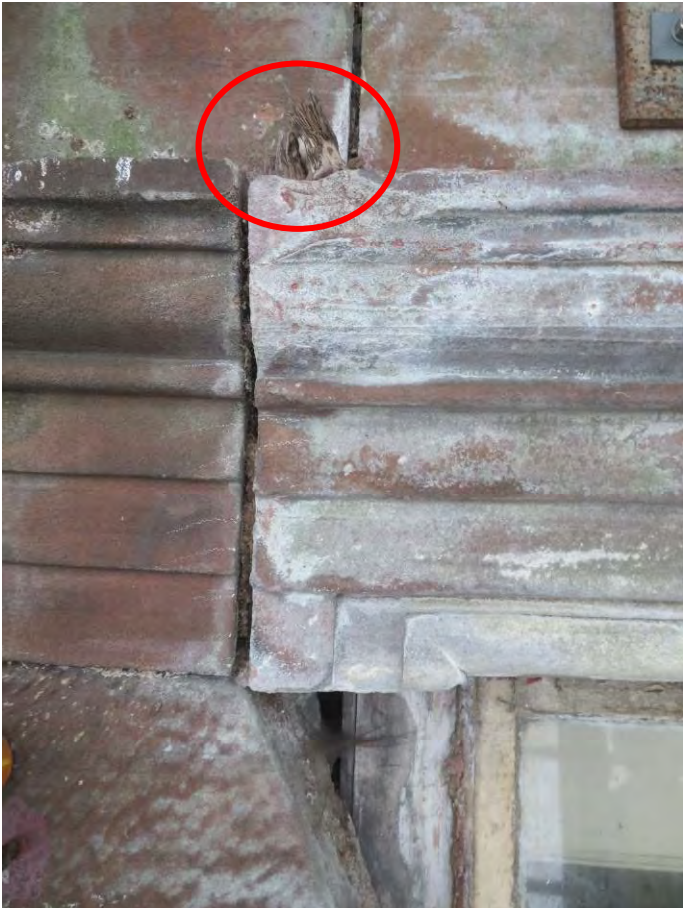
Photograph 48: Root expansion causing fracture
