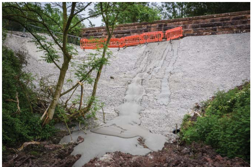
The masonry arch bridge at Great Musgrave, Cumbria, before and after infilling with hundreds of tonnes of aggregate and concrete by National Highways in May 2021 (Credit: The HRE Group)
