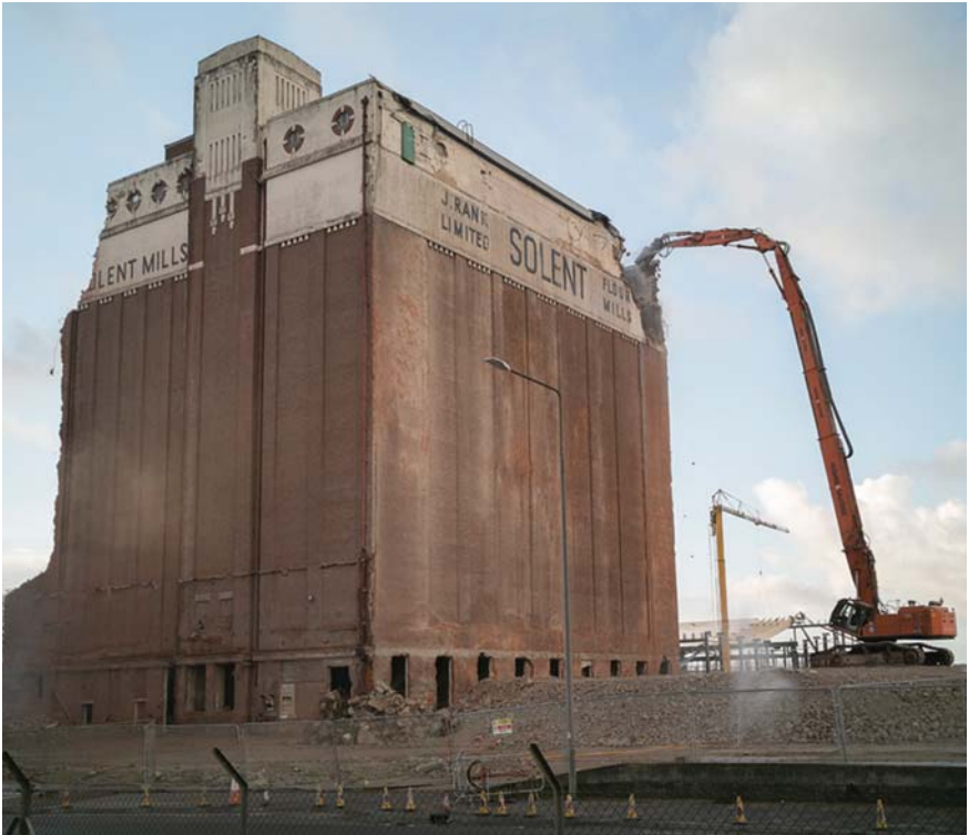
Applicants often make proud claims that the vast amount of waste materials from demolitions such as this – the Art Deco Solent Flour Mills in 2020 – will be majority recycled. Sadly the reality is that materials such as brick, stone and concrete (which make up a vast proportion of construction waste) are recycled by crushing and re-using as aggregate and hardcore for roads (Credit: SBH)
